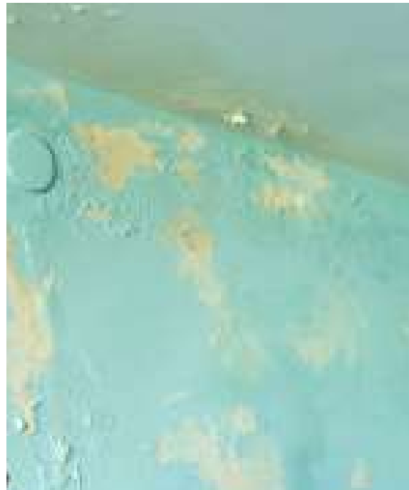
The wall inside of the 1 st floor (basement floor): the waterproofing of the wall is probably broken or absent, and exhaust ventilation is also absent.
