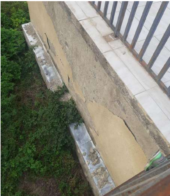
Due to the lack of a roof, the walls are not protected from water, the plaster falls off. And there is no blind area (protective paving) around the house
