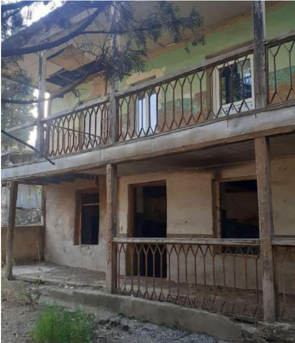
The Multifunctional Community Center with the library on the 2 nd floor. Room on the 1 st floor is empty, without windows, needs remon.
