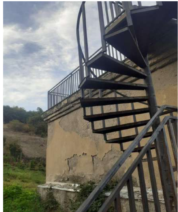
The metal staircase to the terrace and the wall of the 2 nd floor
